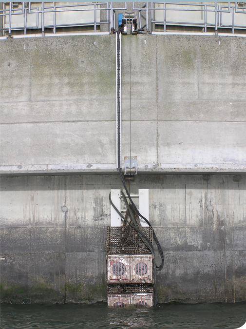
Detail of winch system used for deploying Sound Projectors
