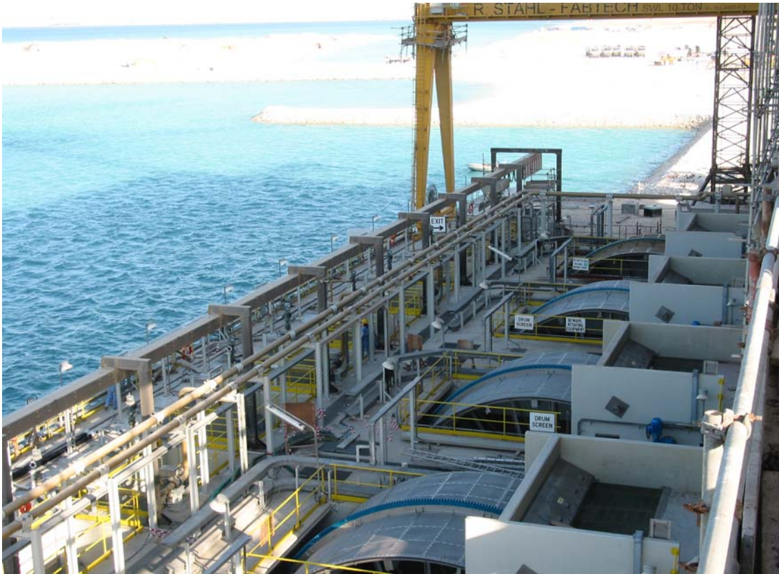
Figure 5-9 Overhead view of typical set of four drum screens at a coastal plant
