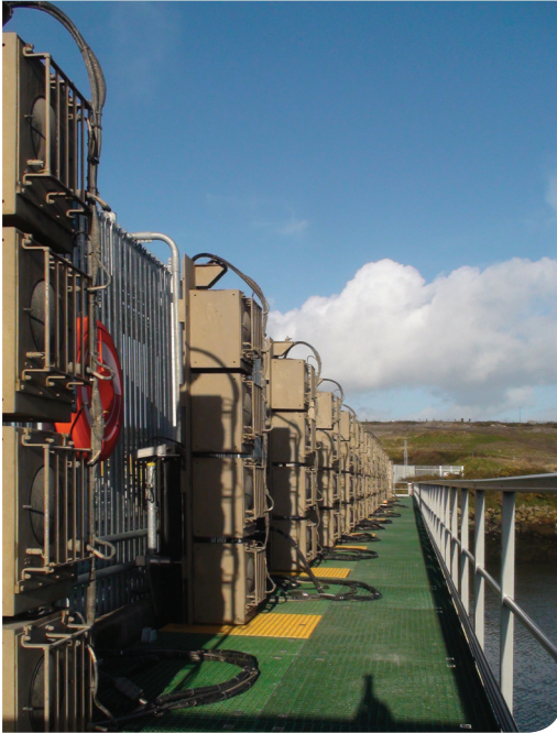
FGS MkIII SILAS® Sound Projectors at Pembroke Power Station
