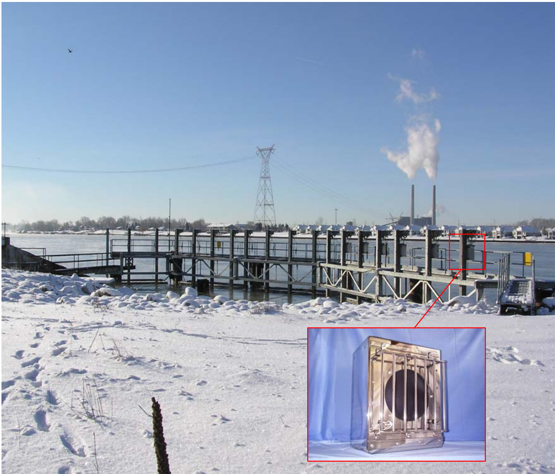
Figure 6-19 Example of an acoustic fish deterrent support structure constructed across a shoreline CW intake at the Lambton Generating Station, St Clairs River, Canada. The vertical beams each act as rails, which allow sound projectors to be raised and lowered for maintenance. The positioning of the structure ahead of the intake opening ensures that the fish repulsion zone is in an area of low water velocities from which the fish can escape. The inset shows an individual sound projector. (Main photo courtesy Paul Patrick, Kinectrics).
