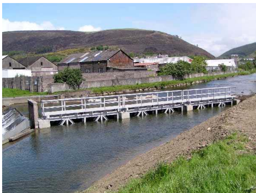
Plate 3.1 Fixed panel screen installed on the R. Afan, Port Talbot in 2003, to prevent salmonid smolts from entering the docks feeder.
