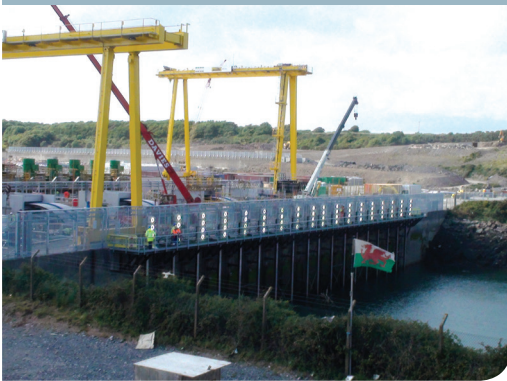
FGS SILAS® System installed at Pembroke Power Station
